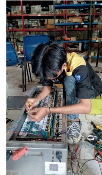
Proses Pembuatan battery LiFePo4 10kWh, 96Vdc
